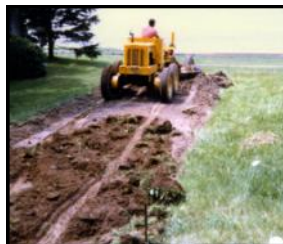
We became contractors and hired heavy equipment operators, electricians, plumbers, carpenters, and various tradesmen to complete the project.
